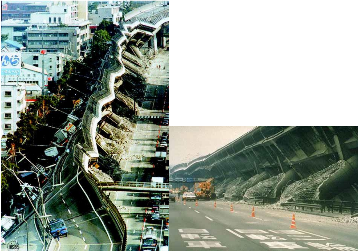
Figure 14: Base shear failure in the 1995 Kobe Earthquake
